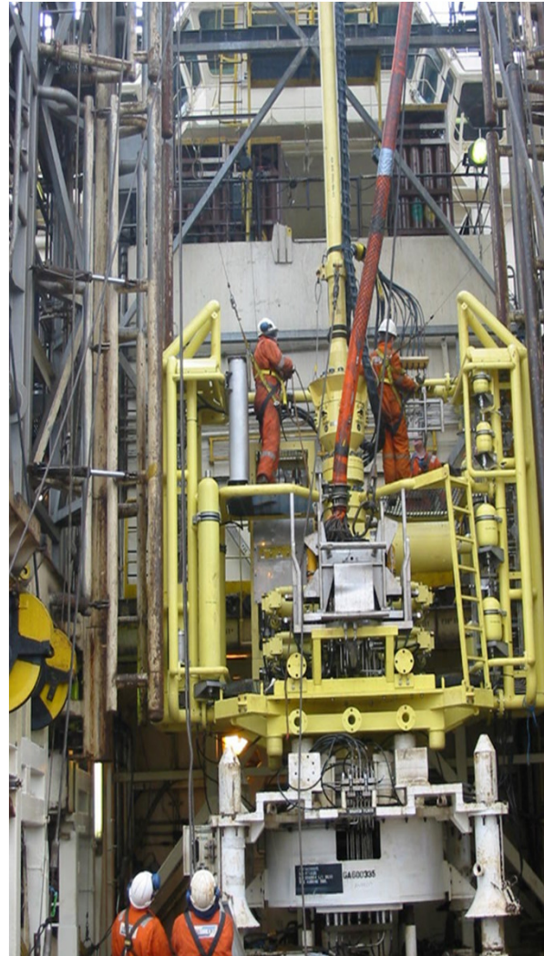
5 1/8" SIL in the MSV Seawell Derrick
